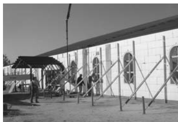
STEEL STUDS & TURNBUCKLES
